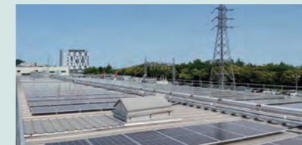
Solar power generation equipment installed on the roof of the Isohara Works
