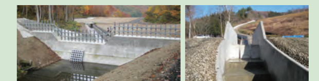
Countermeasure construction: Installation of check dams (driftwood stopper) Countermeasure construction: Upgrading drainage channels
