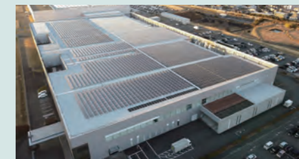
Solar power generation equipment installed on the roof of the Kakegawa Works
