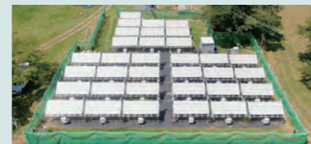
Test plant for artificial photosynthesis technology (courtesy of ARPCChem)
