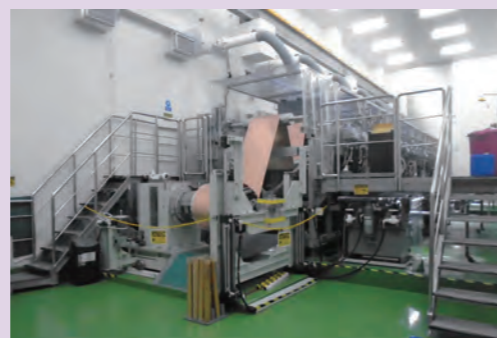
Facilities for treated rolled copper foil surface treatment
