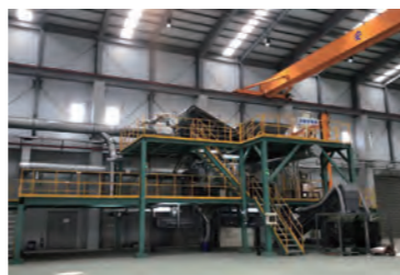
New crusher and automatic sampling equipment
